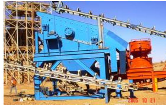
VIBRATING SCREEN 6 'X 16' AND CONVEYOR BELT IN LA HERRADURA
