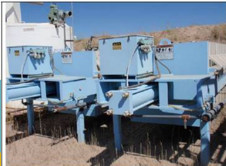
Filter Presses. Two each. Each press is 19' long and 5' wide
